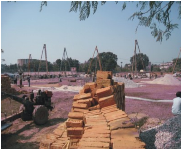
A view of Bheramara rental power site. Its works have begun before contract signing.
